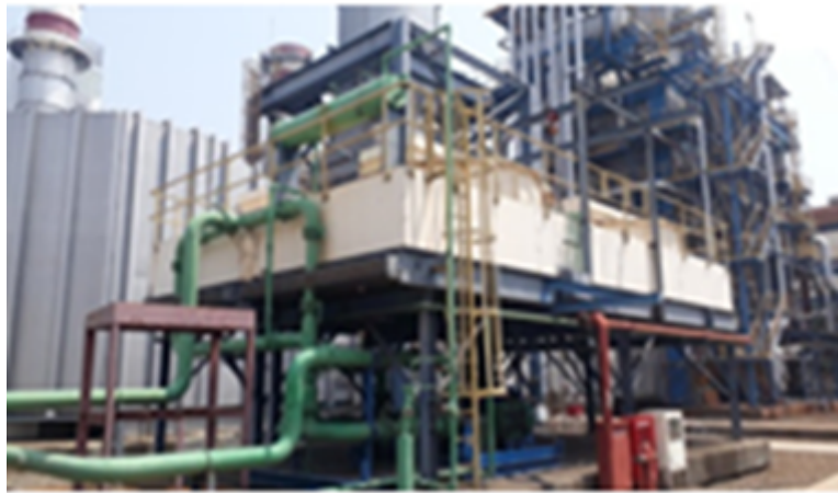
Figure 1. Radiator turbin gas PLTGU PT. PJB UP. MuaraKarang Blok 1
